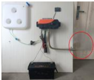
Excessive pump oil produces white smoke
