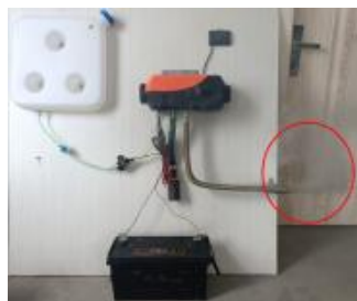
Excessive pump oil produces white smoke
